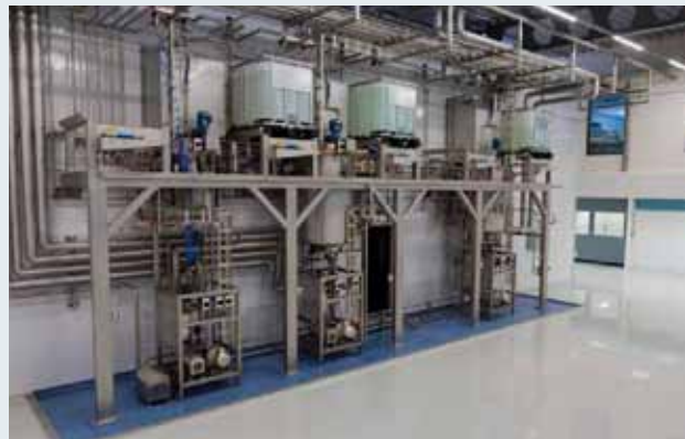
Figure 5: Process vessels and stacked raw material containers at 1st floor level in not classified basic hygiene zone as back side of Figure 5.
