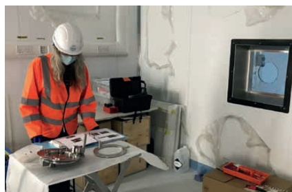
A fluid transfer port being prepared for assembly into its special window in the cleanroom wall panel on the right of the picture
